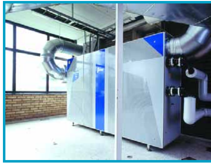
Fig.5: Turbec T100 installed in a boiler room (by courtesy of Turbec)
